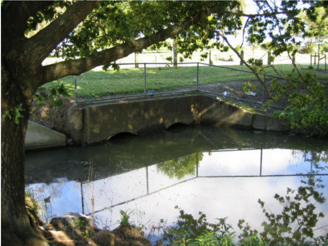
Figure J3: Submerged Outlet to Pt England Pond (Opposite 115 and 117 Elstree Avenue) (December 2003)
