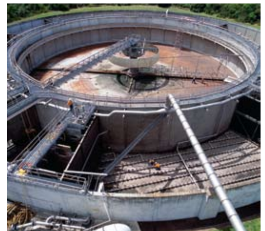
Contractors undertaking routine cleaning and maintenance on 1 of 9 reactor/clarifiers at the Mangere Wastewater Treatment Plant. This circular unit is 77 metres in diameter and can hold 31.3 million litres of effluent.
