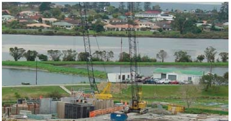
Early construction of the now completed and operational Orewa wastewater pumping station and storage facility.
