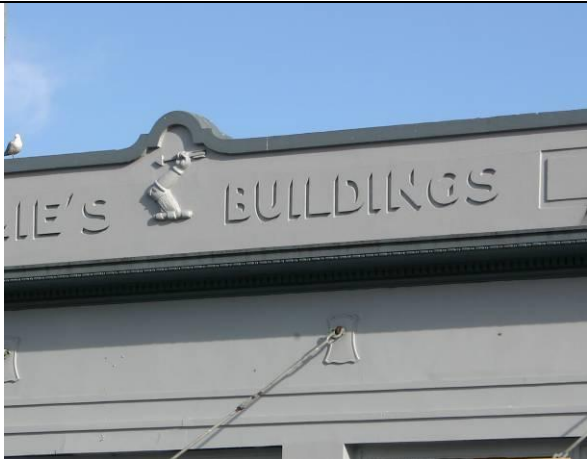
Detail of raised plaster lettering to parapet and arm holding an arrow.
