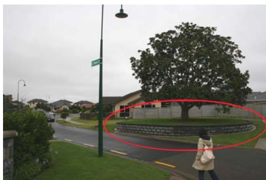
An example of a poor relationship with existing land required to be supported by a retaining wall at Flat Bush.
