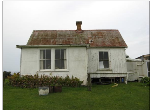
Fig 19: West elevation part re-clad in fibrolite. The balance is clad in T&G. Photo: Reynolds & Associates
