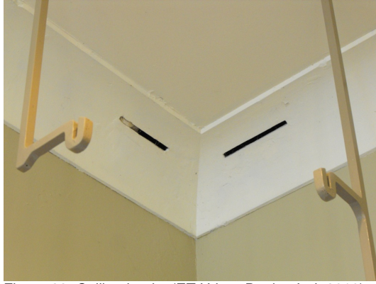
Figure 23: Ceiling hooks (ET Urban Design Ltd, 2010)
