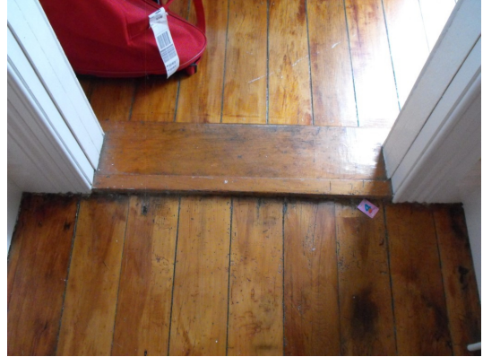
Figure 15: Original flooring (ET Urban Design Ltd, 2010)
