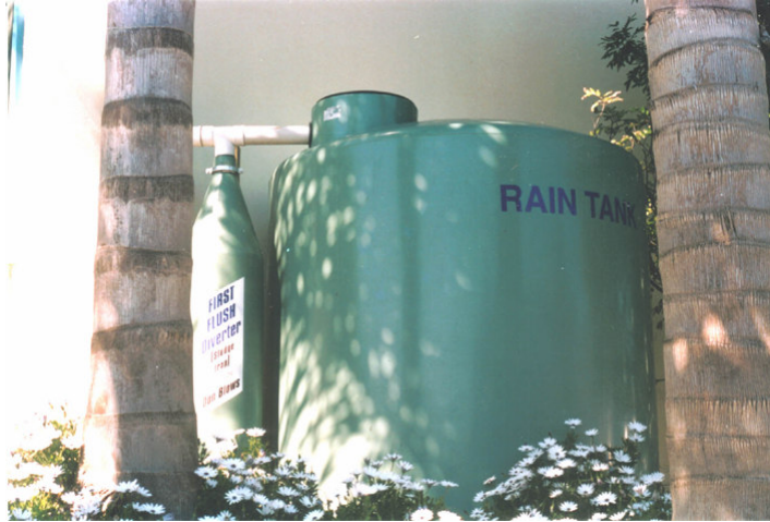
Photo 1 Rain Tank: Plastic Type with First-Flush Diverter
