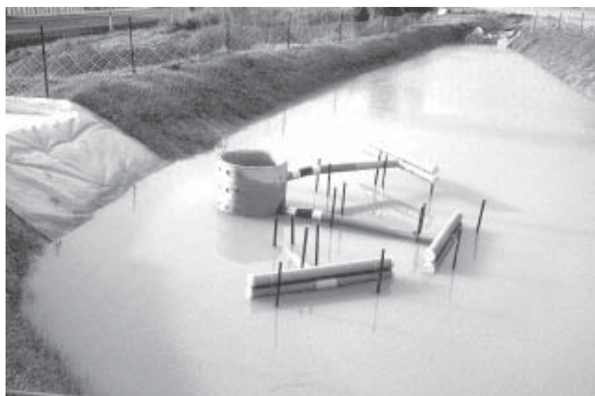
Sediment Pond with Floating Decant
