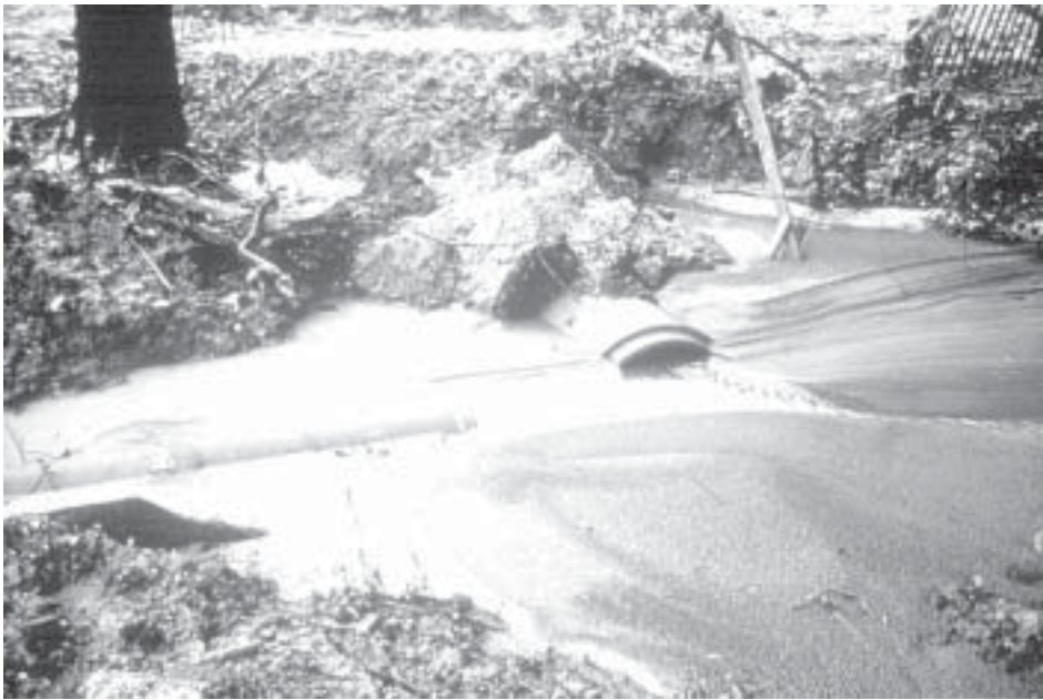
Sediment Choking a Stream Channel from an Uncontrolled Earthworks Activity
