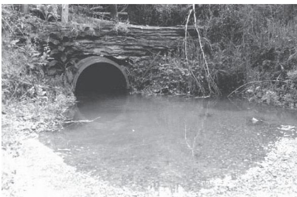
Plate 14: A fish friendly culvert with invert countersunk below the natural streambed.
