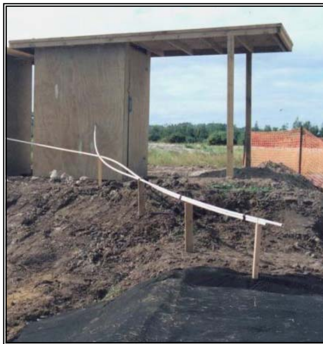
Figure 4. Rainfall Activated Flocculation Housing
