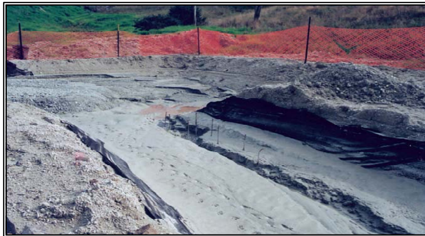
Figure 10: Pond Inlet Channel Full of Sediment
