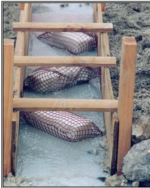
Figure 8: Floc Blocks and Flume Detail
