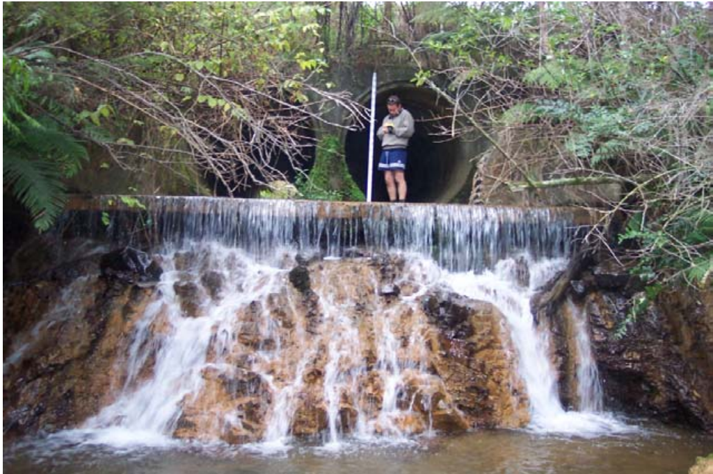
Figure 6: Perched twin culvert the Milne Stream below the Mangatangi Hill Road.
