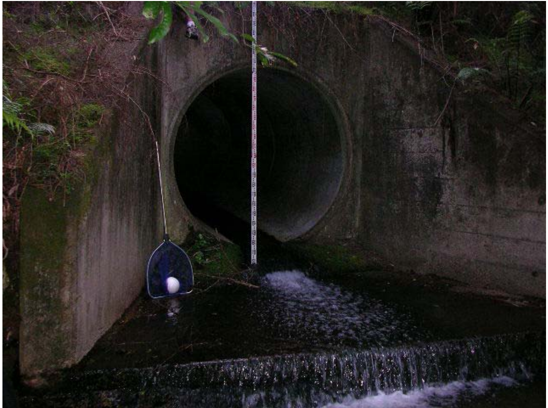
Figure 6: Perched culvert on the Island Stream below the Nihotupu Dam Road. Note both culvert outlet and apron are perched.
