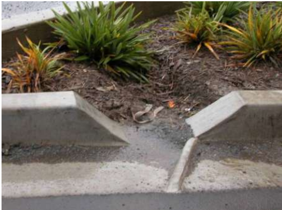
Figure 35 Talbot Park rain garden inlet showing overfilling with soil and mulch, material from adjacent building sites blocking the inlet, and retrofit “wings” to improve entry of run-off (Bracey et al. 2008)
