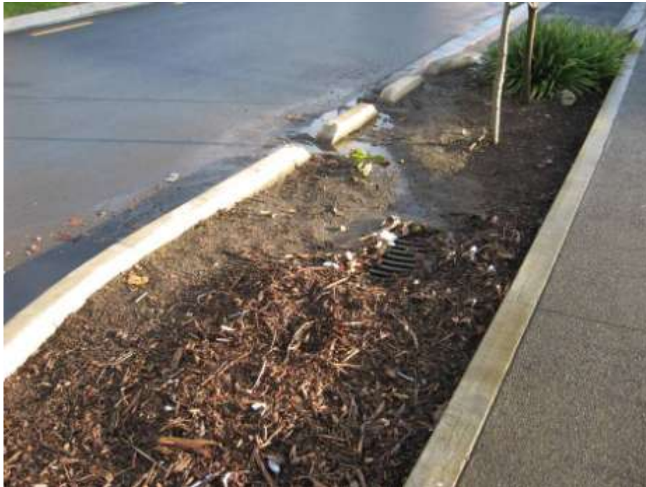
Figure 36 Incorrect soil and mulch levels combined with narrow kerb cuts (Bracey et al. 2008)
