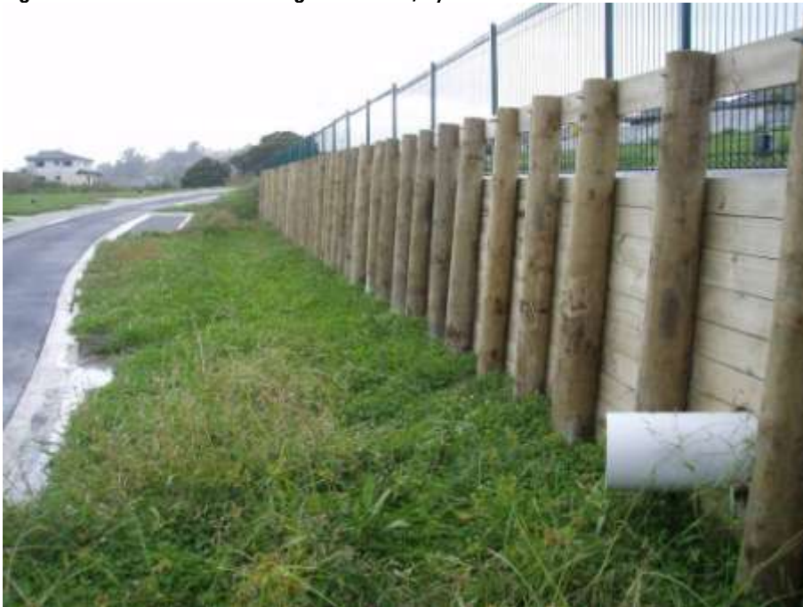
Figure 42 New Zealand Housing Foundation, Pyramid Place: swale
