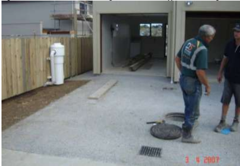
Figure 49 Sonoma Crescent underground rain tanks: type 1 tank arrangement
