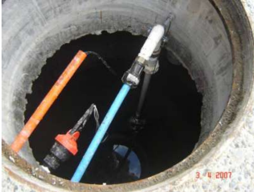
Figure 51 Sonoma Crescent underground rain tanks: tank and pump arrangement
