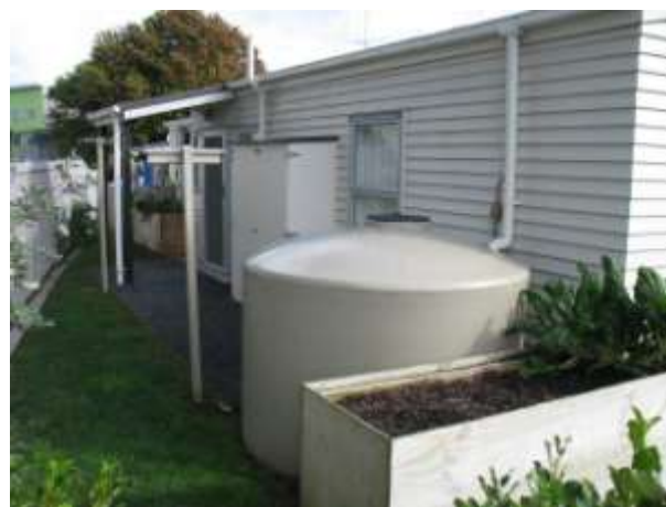
Figure 11: Individual dwelling rain tank at Talbot Park
