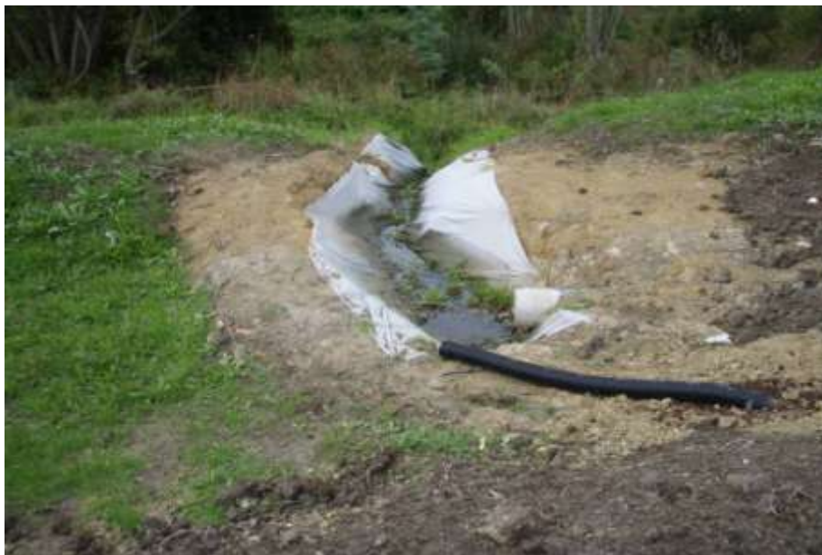
Figure 44 New Zealand Housing Foundation, Albionvale: temporary flow diversion at head of swale
