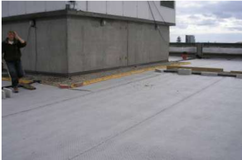
Figure 22 A drainage mat was installed on the roof prior to the addition of soil media
